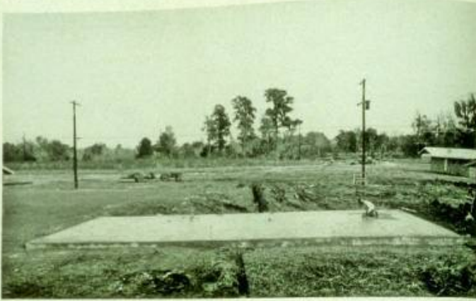
FINISHED SLAB awaits framing crew. This construction is set in 14-day building schedule.
